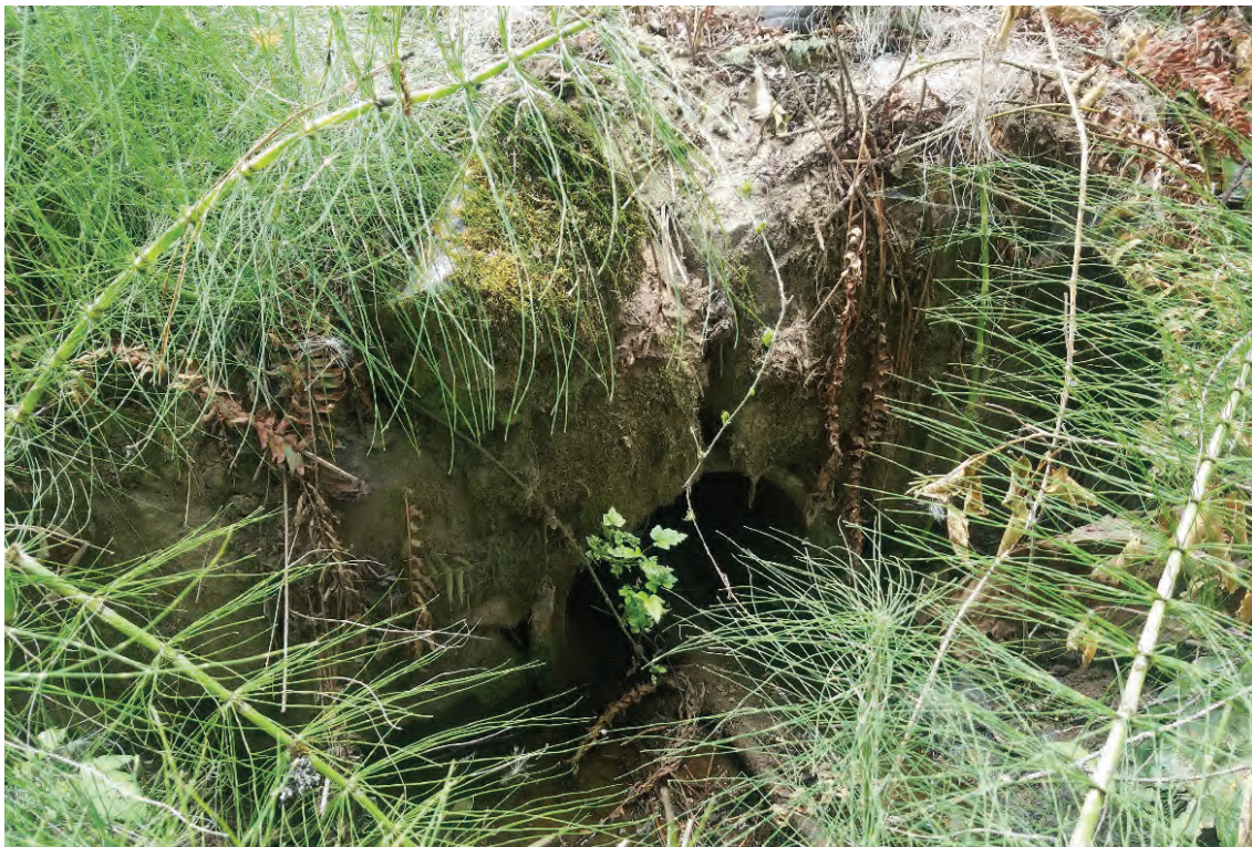
Figure 10: Culvert is undersized and is a barrier to wildlife passage.
