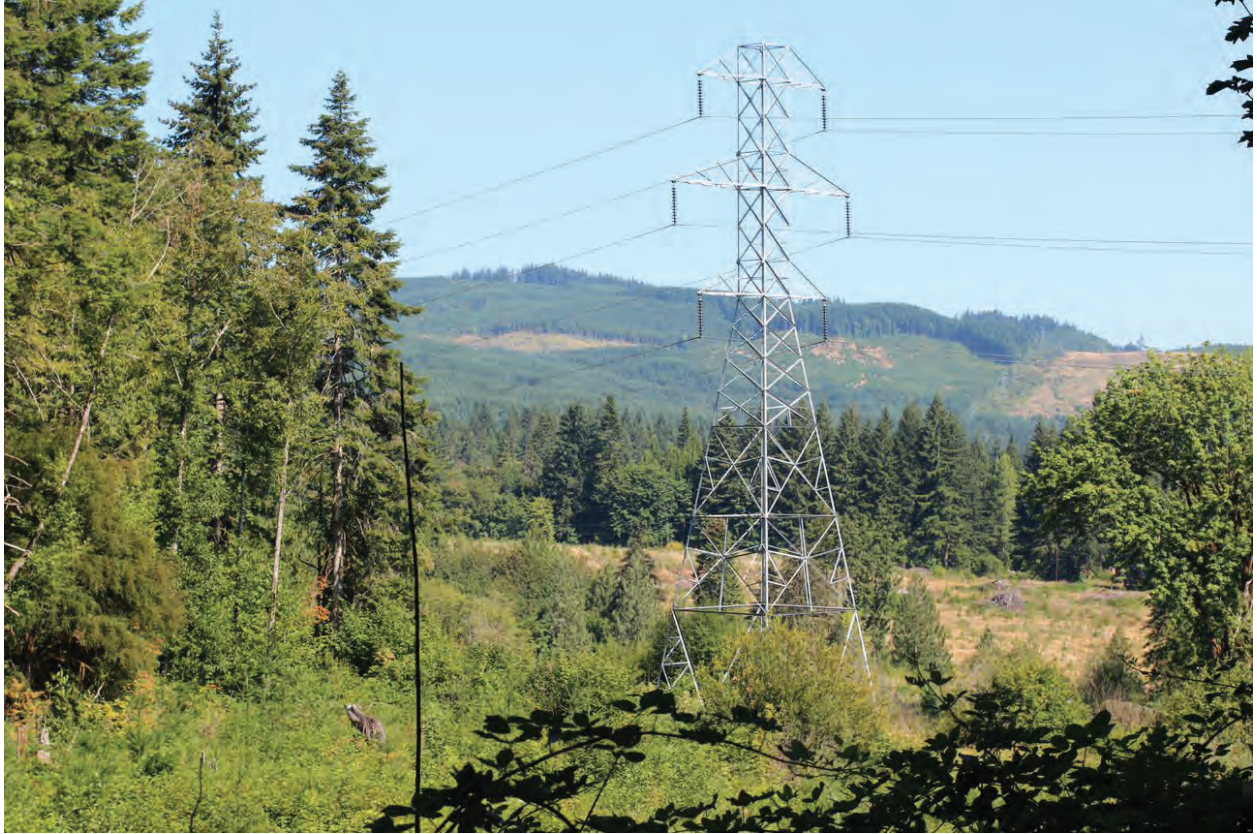
Figure 2: BPA easement for high voltage powerlines near the unincorporated community of Holbrook.
